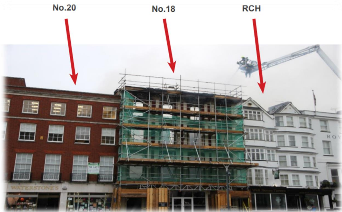
Figure 9 - View from Cathedral Green (Post internal collapse of No.18)
